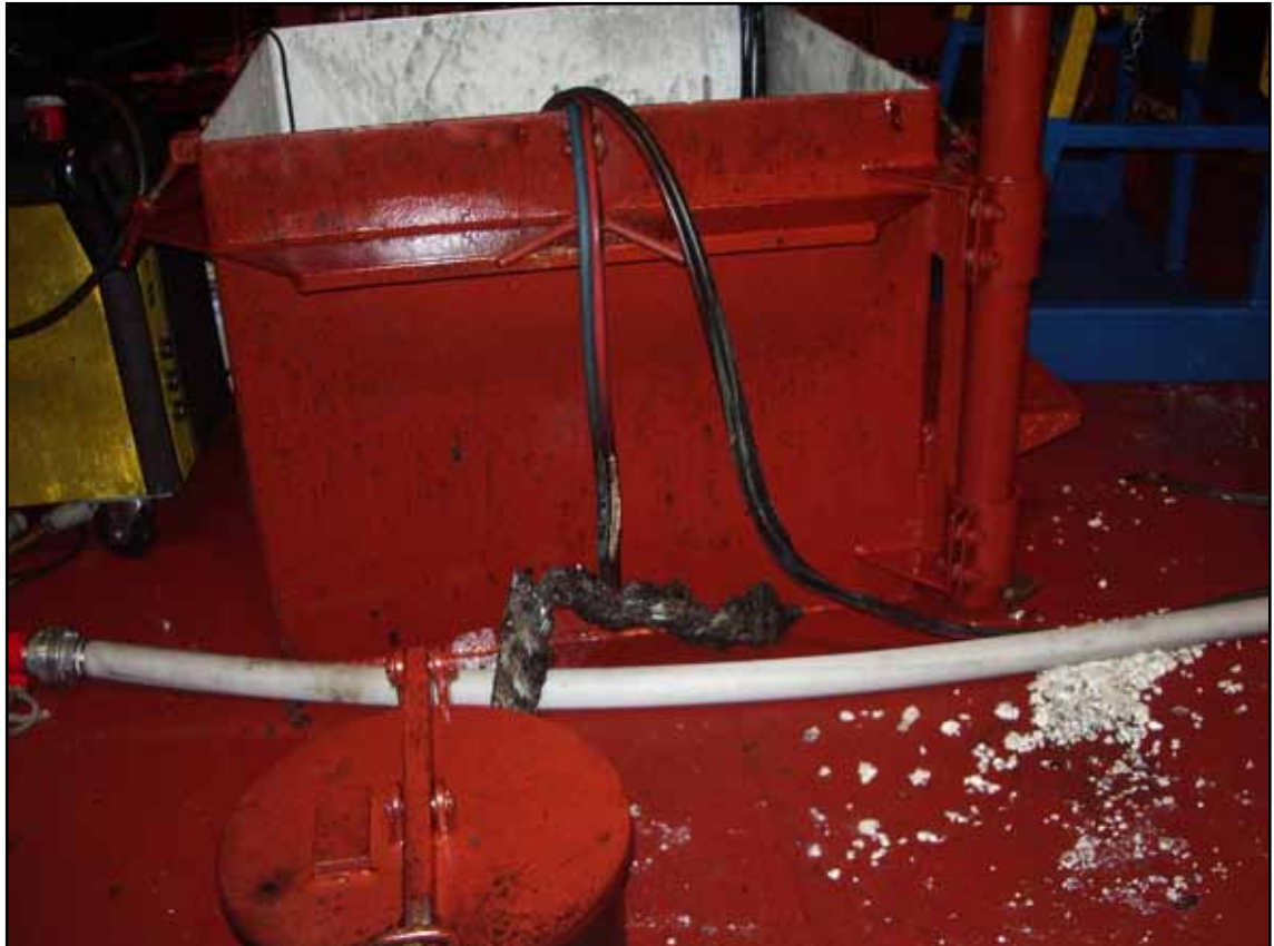
Acetylene and oxygen hose fire damage
