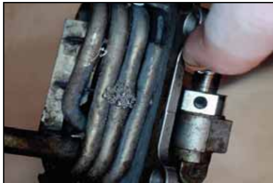
Photo No. 5: Sensing tube leak
