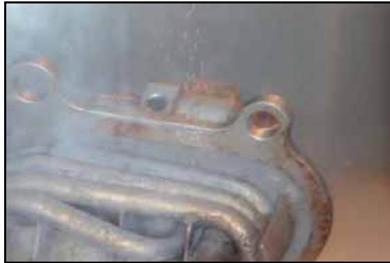
Photo No. 4: Sensing tube leak
